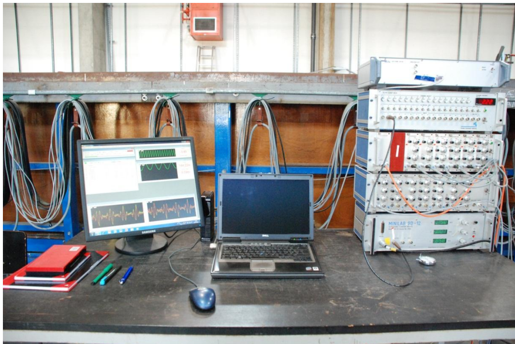
Figure 5.6 DHI's data acquisitions system.
